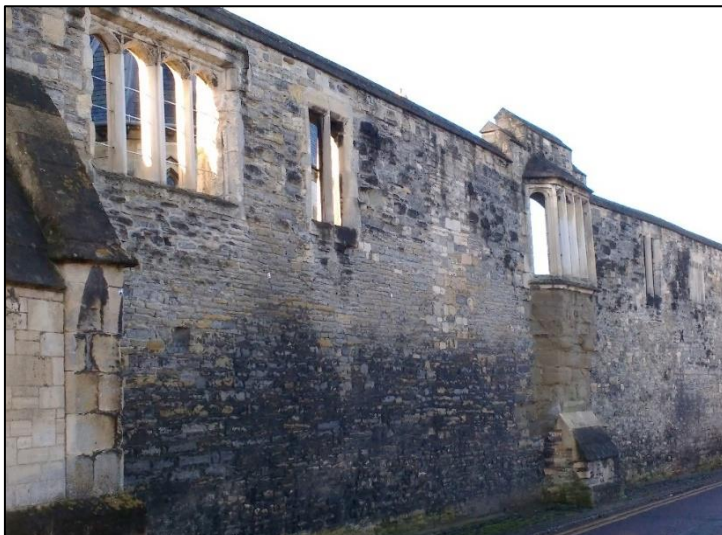
The remains of this gallery wall and its windows, which overlook Pitt Street, are shown in this picture.
